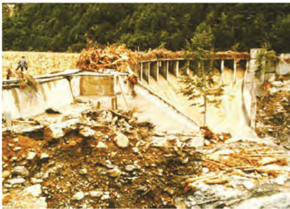
Fig 1: Blocking of spillway at Palagnedra Dam in 1978 (Photo: Ofima SA).
