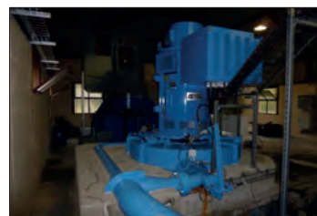
Figure 4. Picture of a Pelton turbine with two injectors from the power plant Le Lauzet in France (Cerec Engineering):
