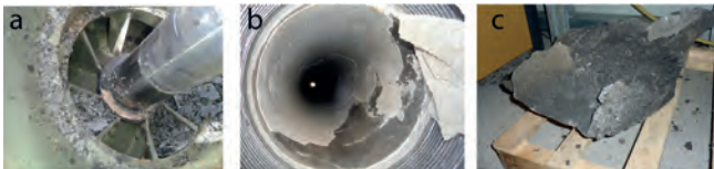
Fig. 2: Scales formed along (a) the pump, (b) the riser pipe, and (c) in installations of the geothermal plant at the surface.
