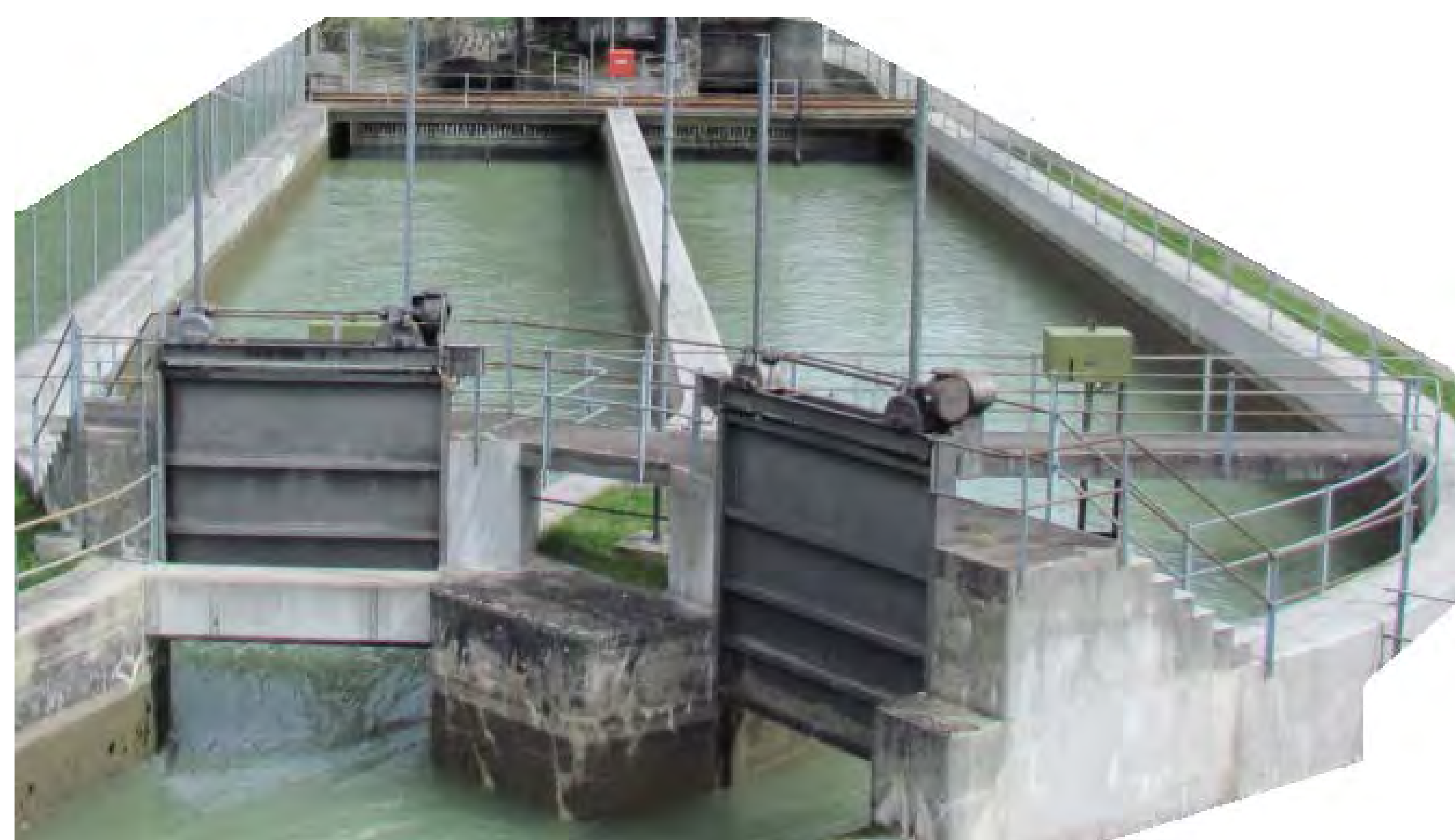
Figure 1 Desanding facility Mörel (hydroelectric power plant Massaboden)
