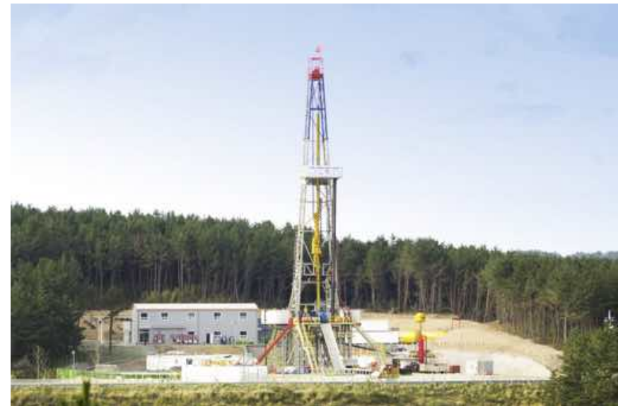
Drilling rig on project site in Pohang/ South Korea (source: DESTRESS Project)
